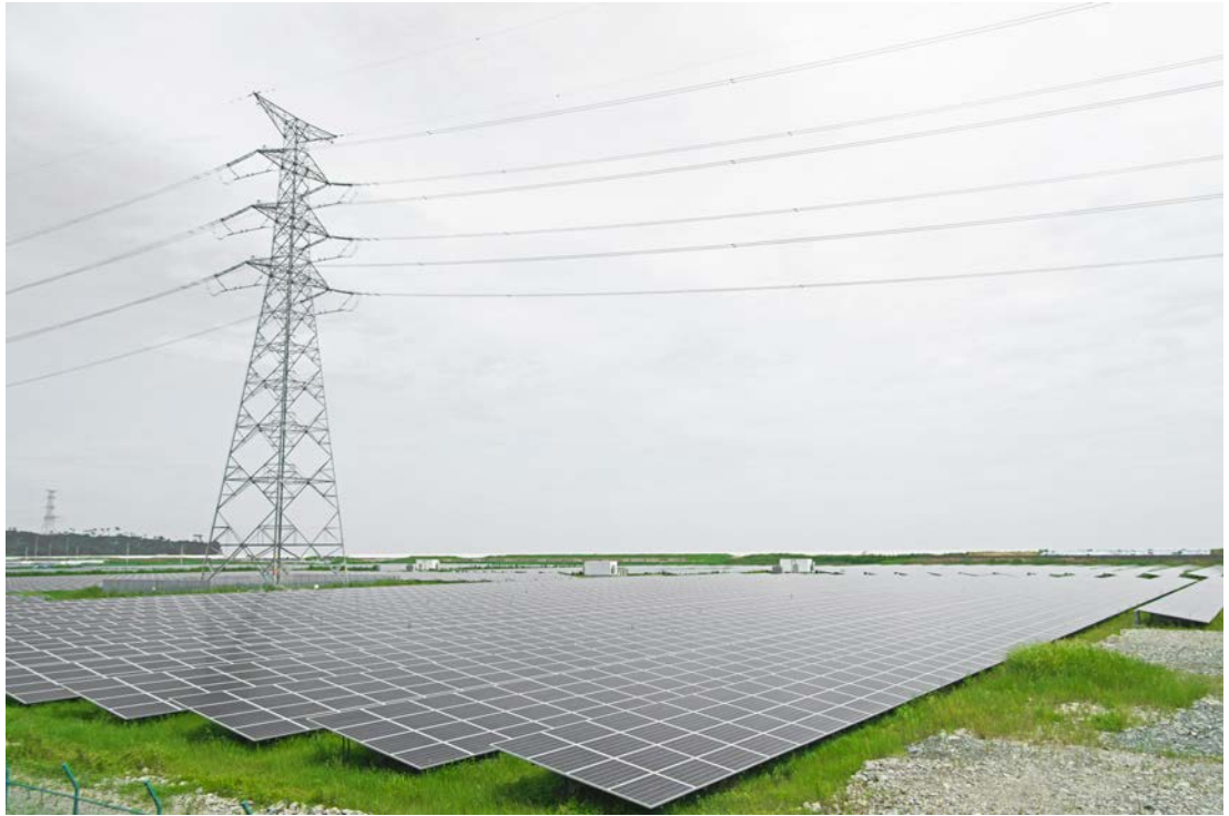
Japan; Minamisona photovoltaic power plant | Gettyimages
