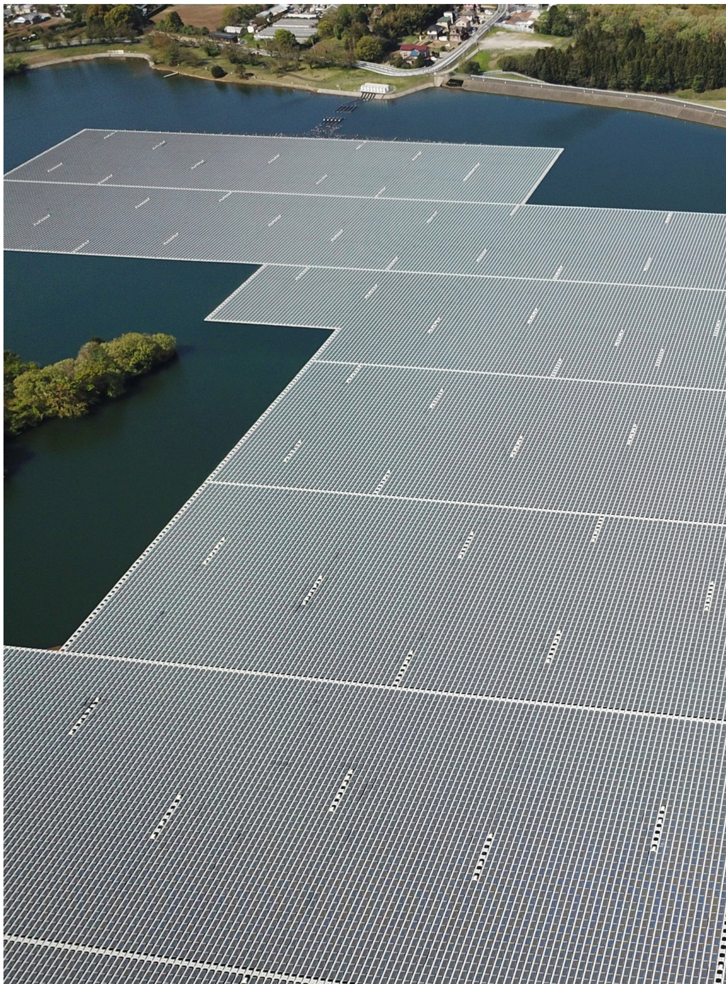
Floating solar power plants, Jamakura dam, Japan | Gettyimages
