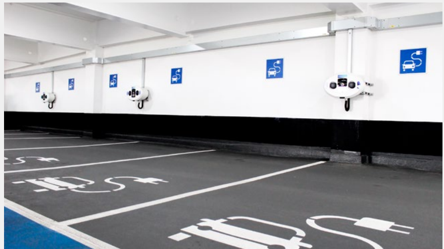
To meet the anticipated growth in EV usage, significant investments in charging infrastructure will be needed
